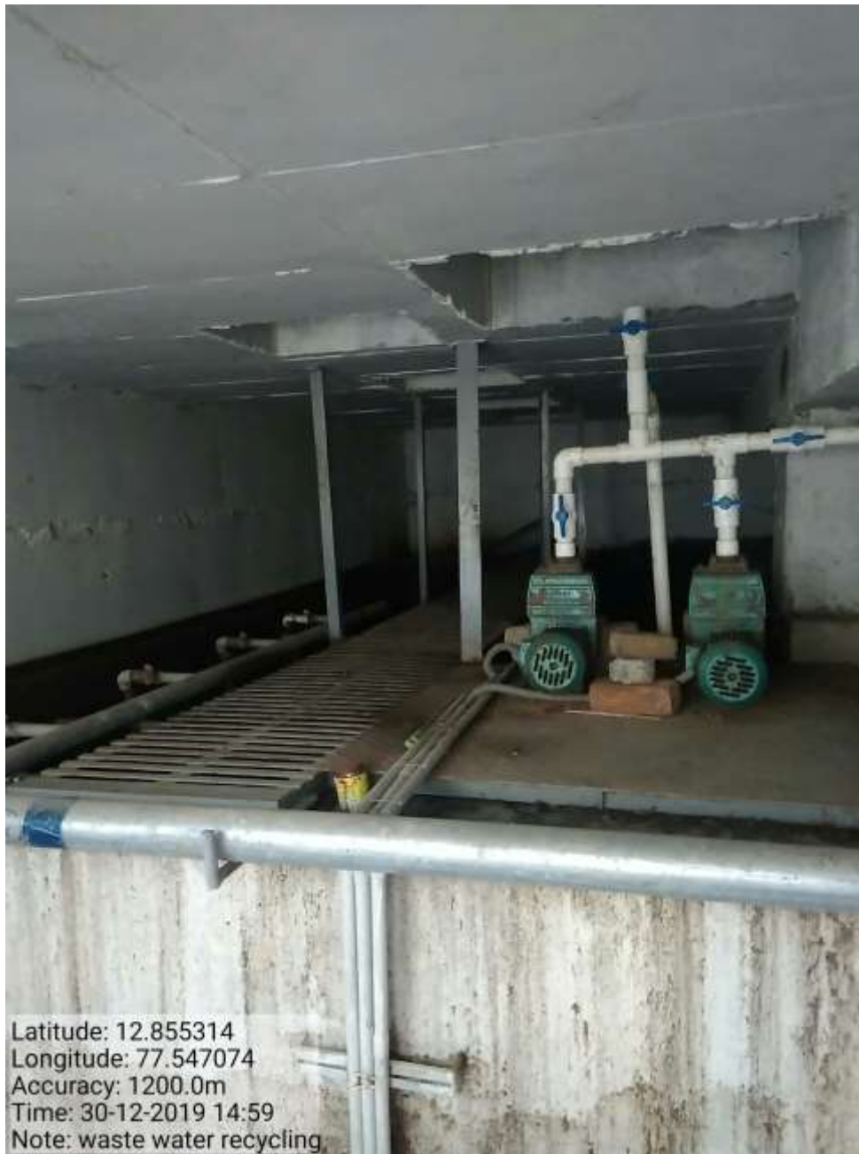
Waste water recycling plant
