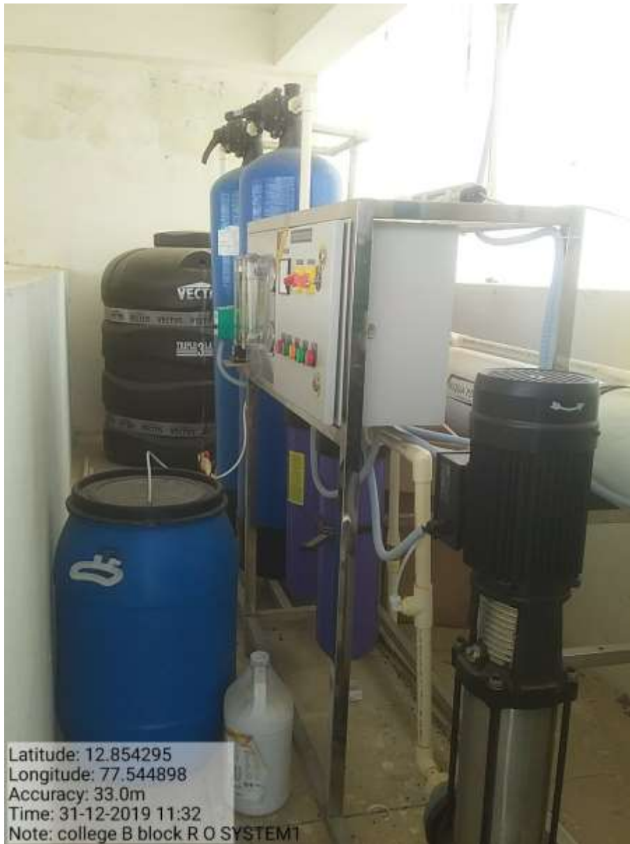
B BLOCK RO SYSTEM
